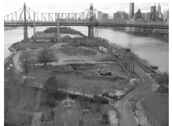
The Southtown construction site as it appeared Thursday afternoon, after the RIOC Board discussed the agency's victory in law suits opposing its layout.
